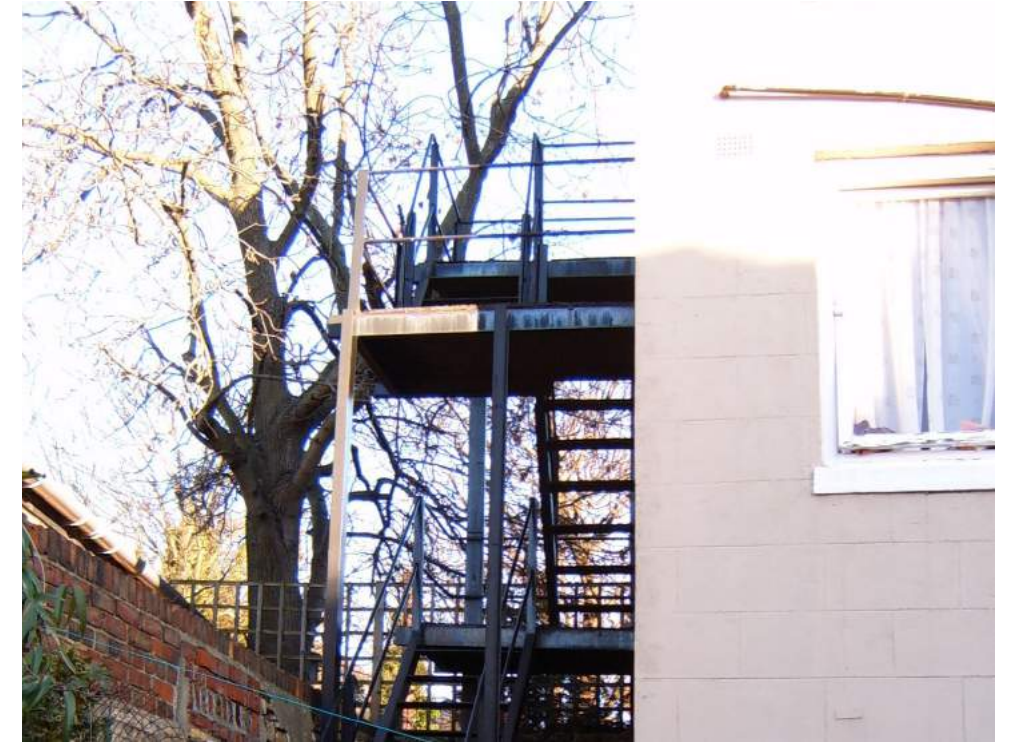
EXISTING STEEL FRAME FIRE ESCAPE LOCATED AT THE REAR OF THE EARLY GEORGIAN TERRACED UNITS
