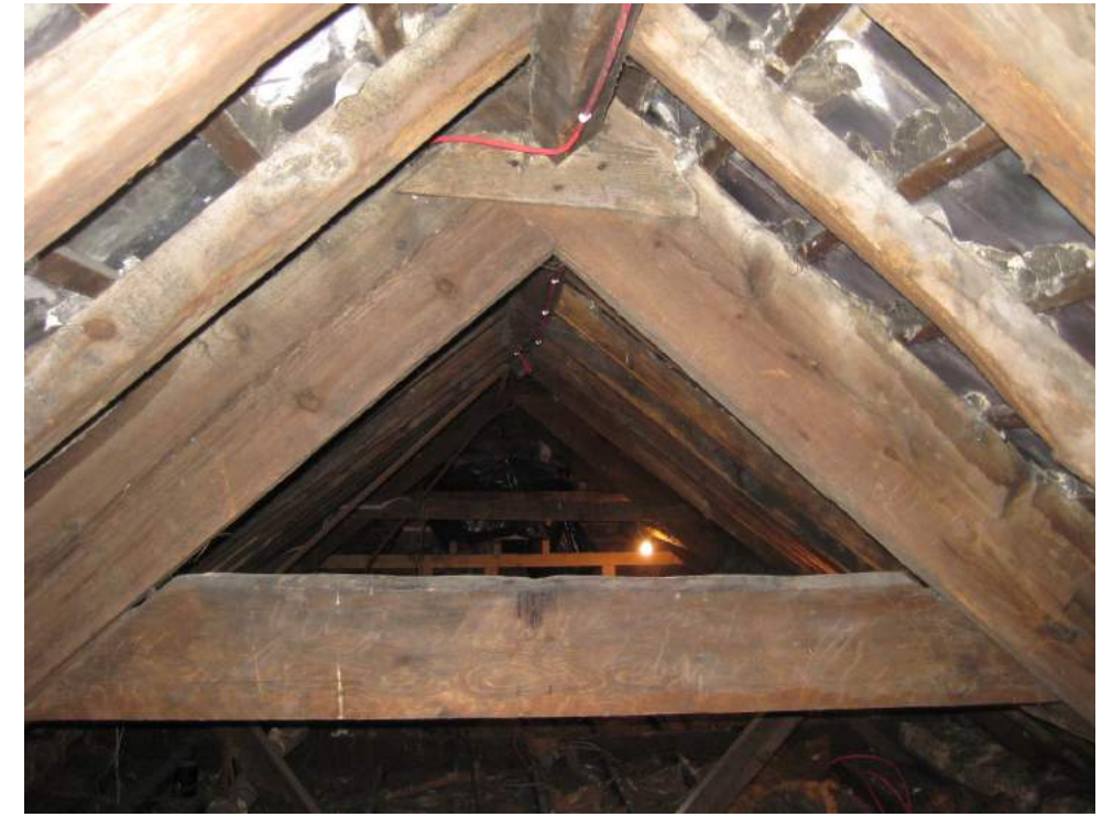
DETAILED VIEW OF THE ROOF STRUCTURE SHOWING THE DISINTEGRATED MORTAR BED TO THE UNDERSIDE OF THE SLATES
